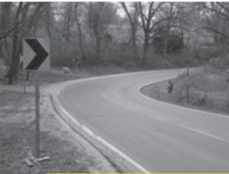
A high friction surface treatment was added to the outside lane of this curve on K5 highway in 2009 in Leavenworth County.
